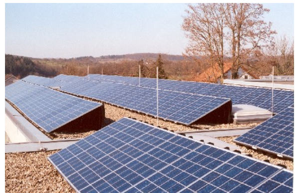
Solar cells for electrical energy production
